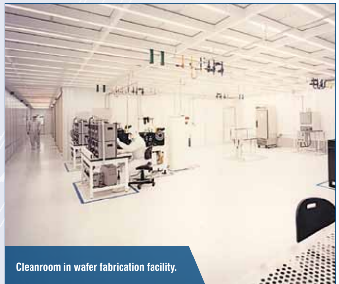
Chase side of a bay and chase cleanroom featuring piping, conduit, and support equipment.
